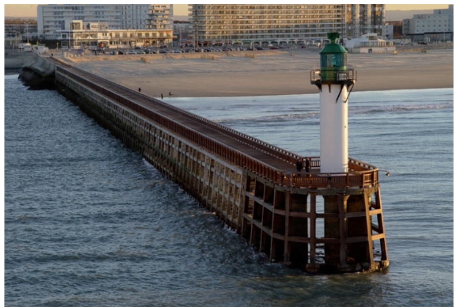
“Tillac” on the Calais pier – Design by Bois et Loisirs(France). Photo D. Delequeuche.
