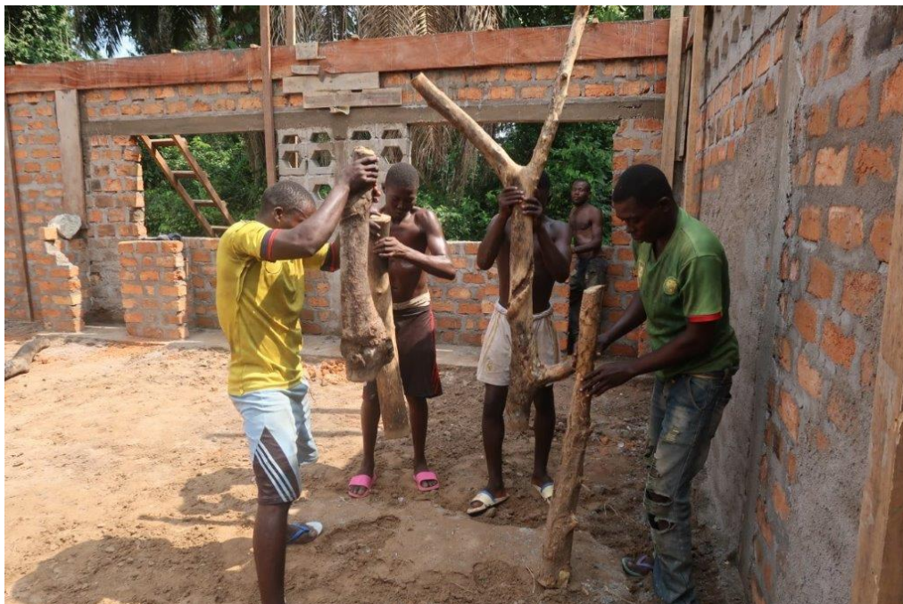
Testing the all-new technology to compact the floor in the new PAPA office © Luis Arranz
