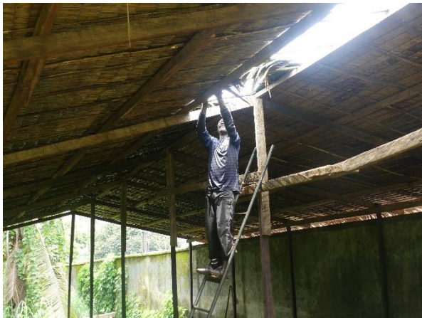
Image 18. Last phase of mat roofing to provide a natural and fresh shelter to the compost.
