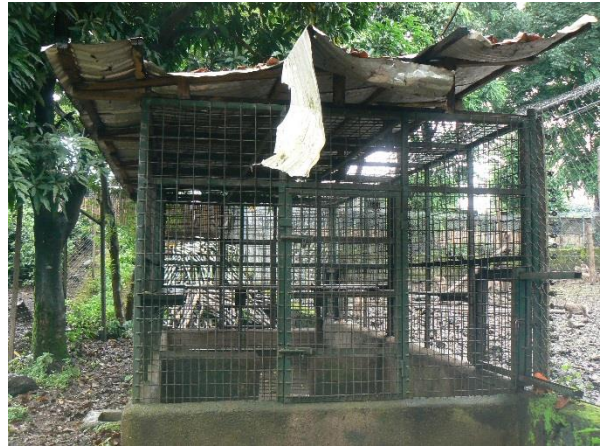
Image 25. View of damage roof of a Drill satellite cage.
