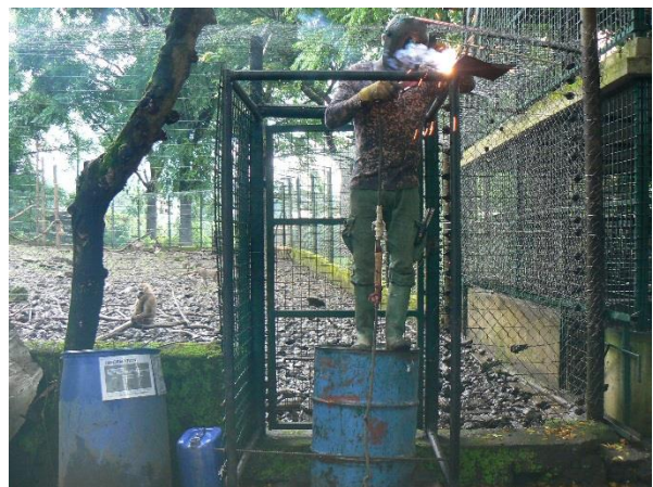
Image 33. Installation of a keeper door to improve the access to the Drill enclosure.
