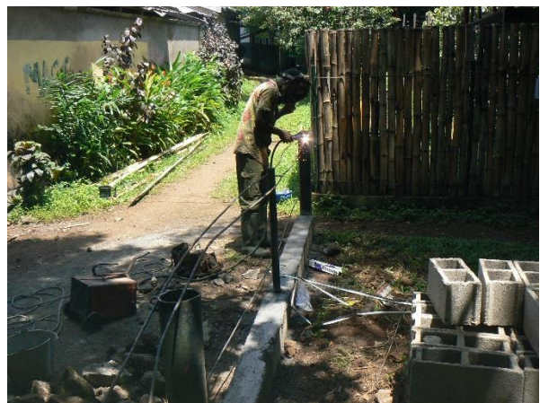
Image 45. Welding of rods on the metal pillar to prepare the bamboo screen in front of the Mandrill enclosure.
