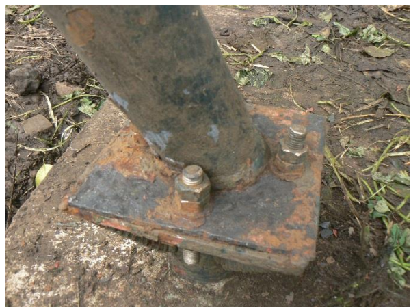
Image 35. Some rusted areas in the Drill metal tree required brushing and painting.
