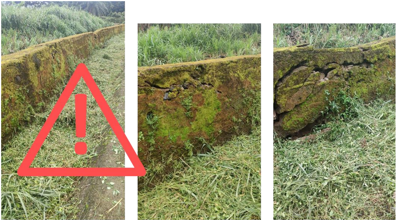
Image 15. The protective wall was built in 2009 to protect the Island of the Limbe Zoological Garden / Limbe Wildlife Centre (LZG/LWC) from flooding and permit the building of animal enclosures. This was necessary to increase the LZG/LWC's husbandry capacity and further support the rescue of victims of wildlife poaching and trafficking in Cameroon. Unfortunately, the lack of maintenance has dangerously weakened the wall that threatens to collapse.
