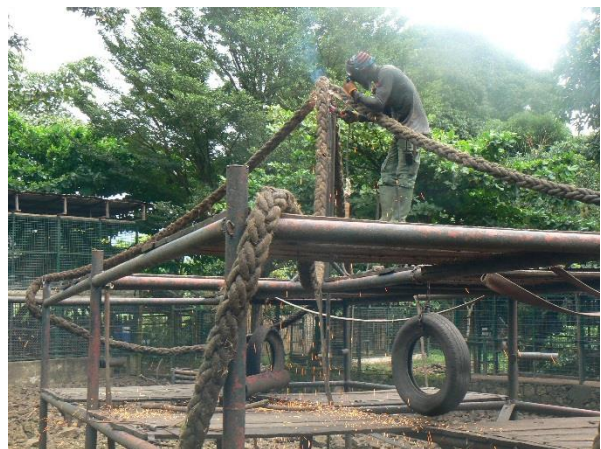
Image 39. Replacing the large rope on the two-level platform in the Drill enclosure.
