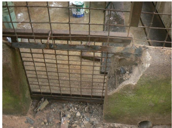
Image 27. Damaged parts of a sliding door in a Drill satellite cage.
