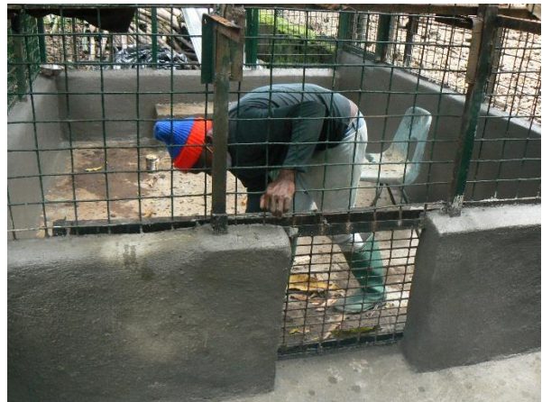
Image 29. Concreting of the floor and wall dressing with cement in a Drill satellite cage.
