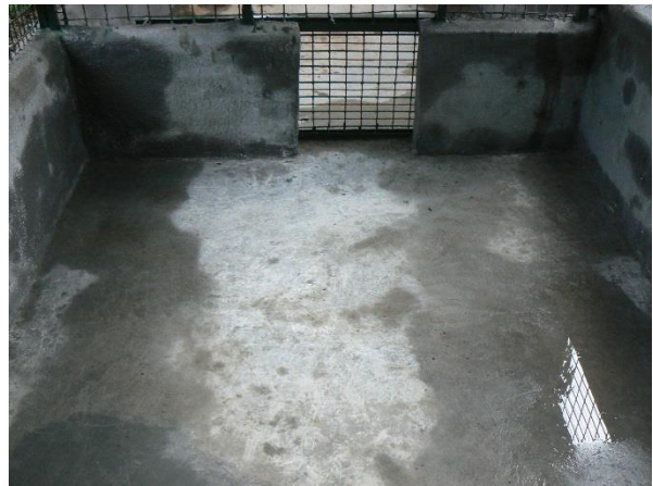
Image 31. The concrete floor is smooth and regular and enables the evacuation of water during cleaning in the Drill satellite cages.
