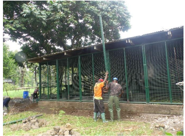
Image 24. Installation of the first metal pole for the splitting of the large gorilla enclosure.
