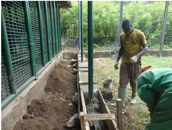
Image 25. Concreting of beam foundation to prepare the splitting of the large gorilla enclosure.
