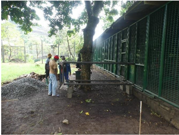
Image 23. Installation and welding of tunnel frame to prepare the splitting of the large gorilla enclosure.
