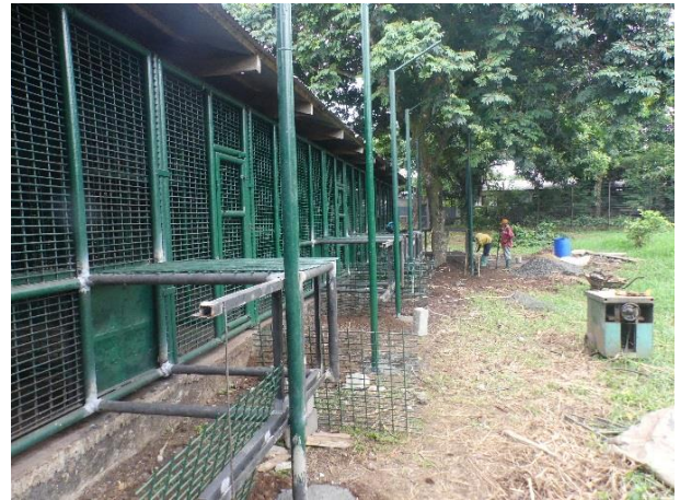
Image 26. Welding of the new tunnel mesh to prepare the splitting of the large gorilla enclosure.
